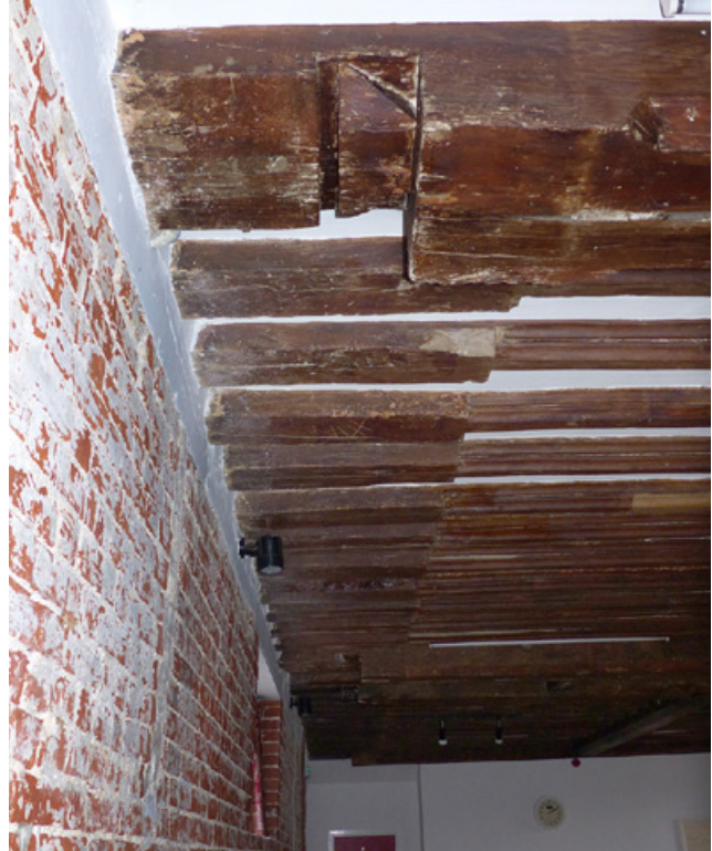
Figure 10: Guildhall GF- east jetty evidence (CAL).
