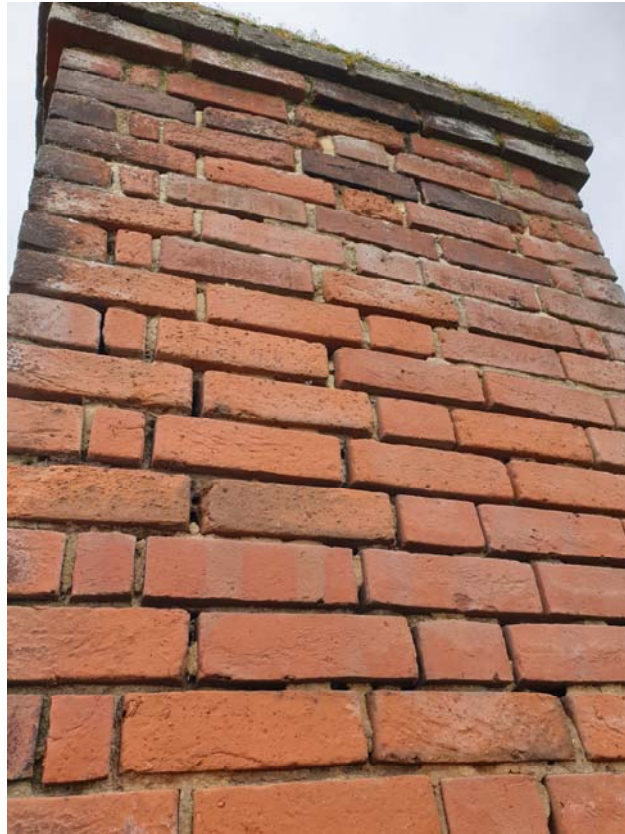
Photograph 21 – Eroded mortar joints to the middle range's chimney
