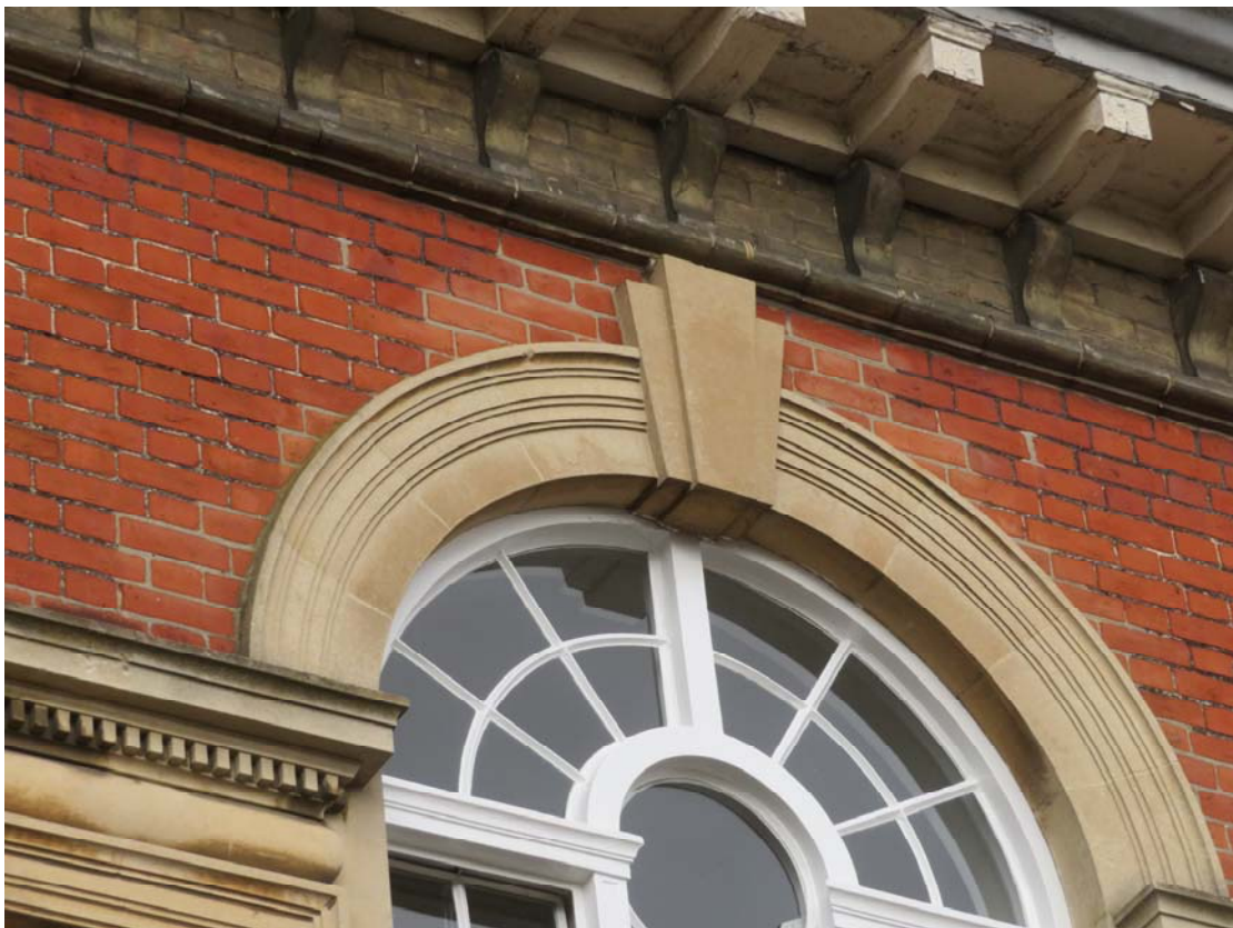
Photograph 120 – Different colour pointing noted to the front elevation
