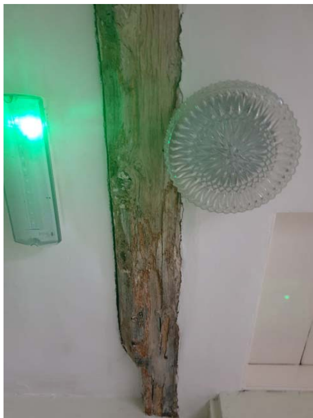
Photograph 62 – Historic wood boring insect attack marks to the beam above 'R3'
