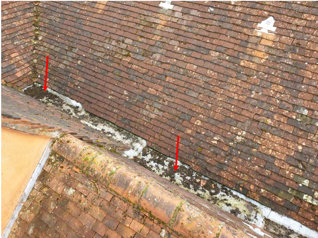
Photograph 04 – Moss and debris build-up noted to the valley gutters
