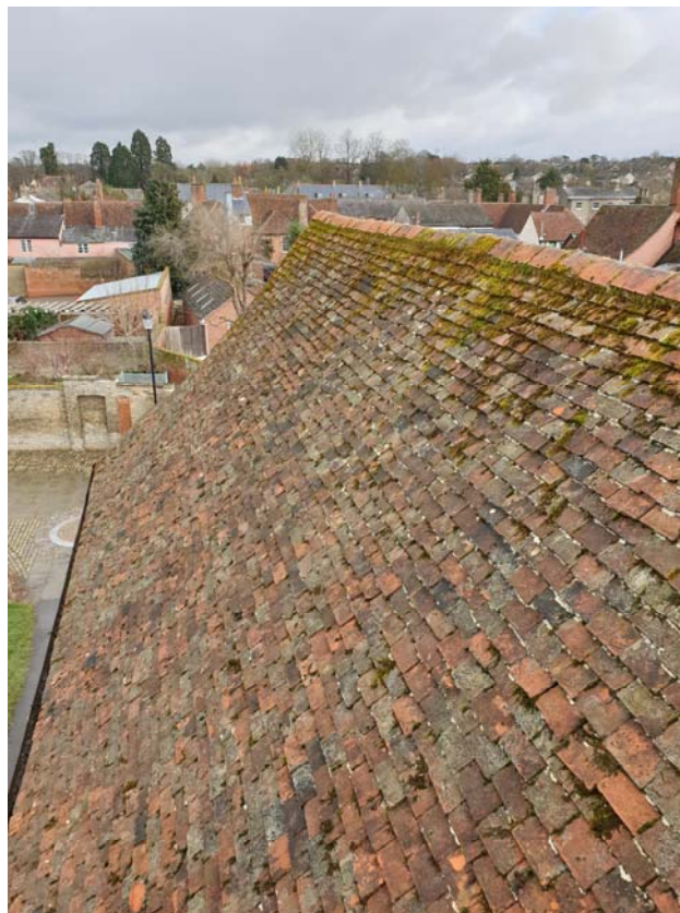
Photograph 42 – Weathered roof coverings (east wing of the Market Hall)
