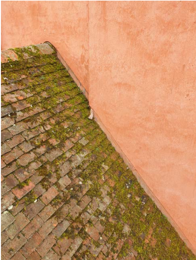
Photograph 43 – Moss vegetation to the west end of the Market Hall’s east range roof
