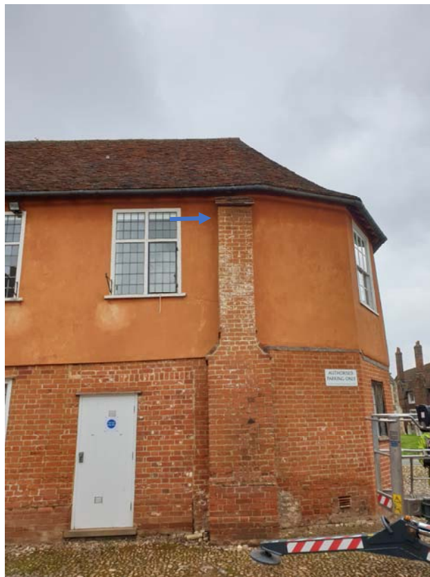
Photograph 48 – Out of plumb brickwork buttress to the south elevation of the east wing
