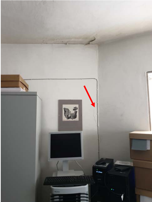
Photograph 74 – Fine crack to the junction of two faces of the brick apse within 'R6' (north side)
