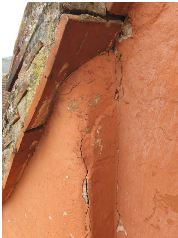
Photograph 26 – Cracking and live render to the east gable of the middle range
