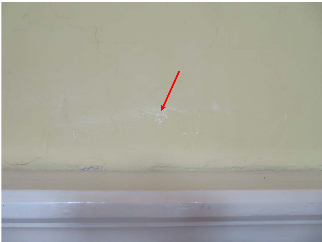
Photograph 138 – Condensation noted to the external wall within the New Town Hall
