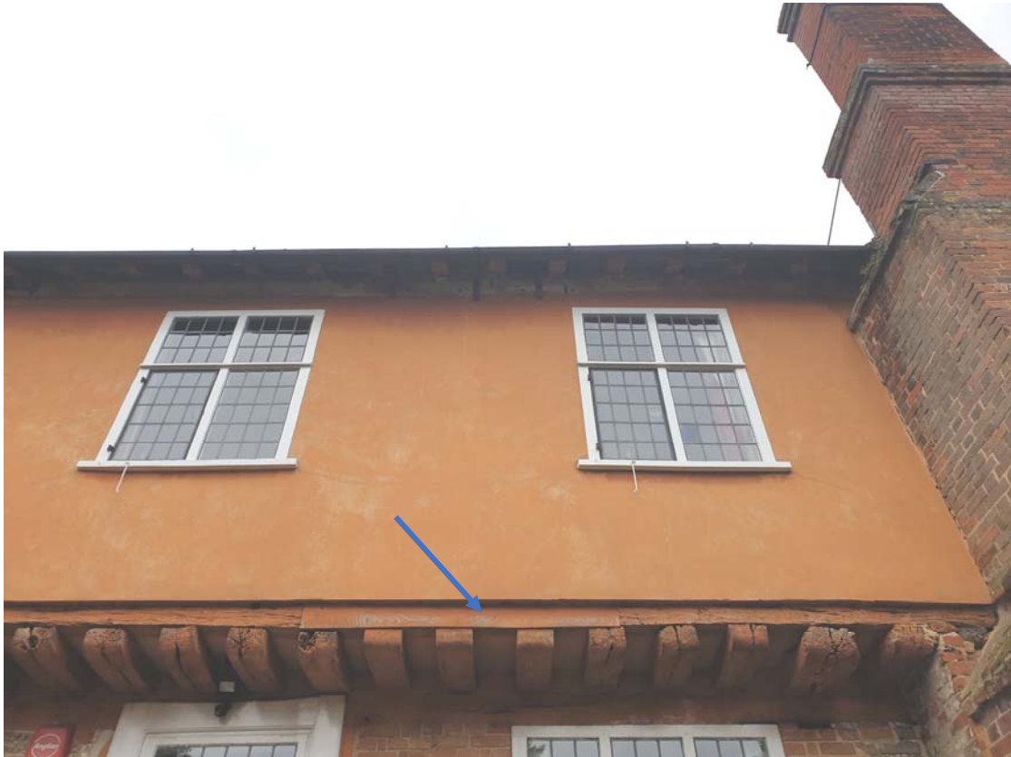
Photograph 96 – Repair to the soleplate of the Old Town Hall's 1 st -floor wall (west elevation)
