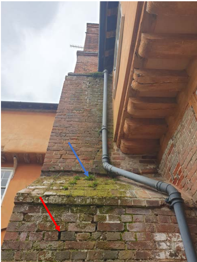
Photograph 94 – Moss vegetation (blue) and eroded mortar joints (red) noted to the Old Town Hall's North chimney (south elevation)
