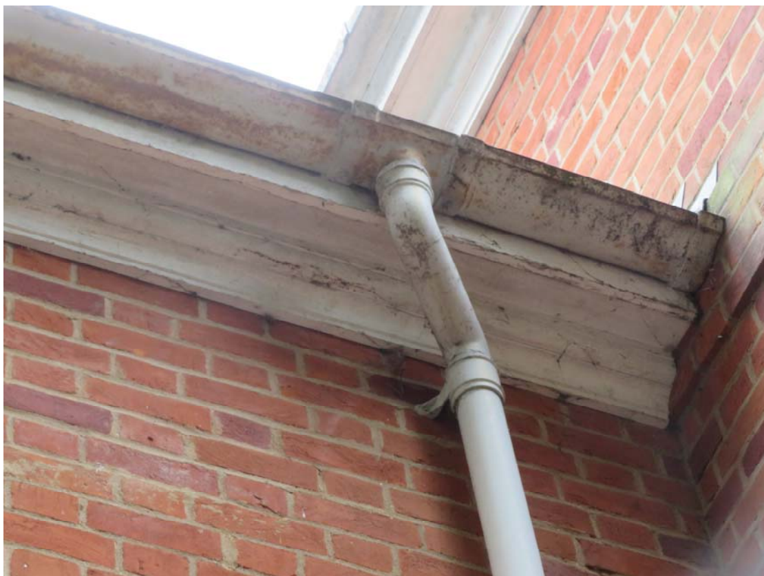
Photograph 126 – Corroding gutters noted to the west elevation of the New Town Hall
