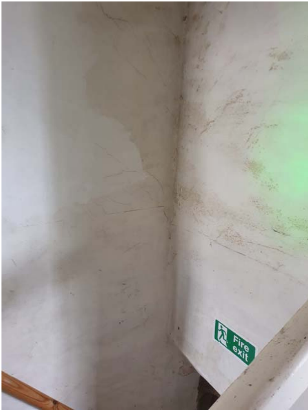
Photograph 54 – Live plaster noted in room 'C2'
