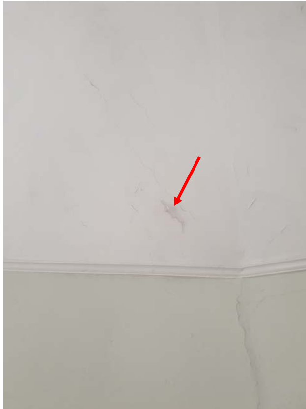
Photograph 67 – Paint flaking off at ceiling level noted in 'R1' (east end)
