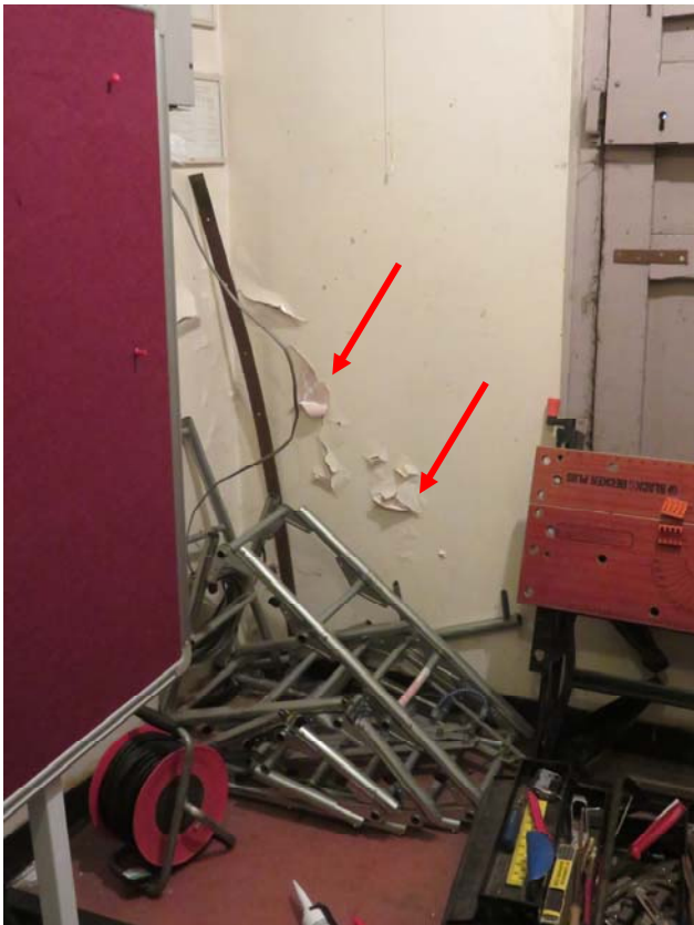
Photograph 140 – Signs of water ingress noted in the service rooms (New Town Hall)
