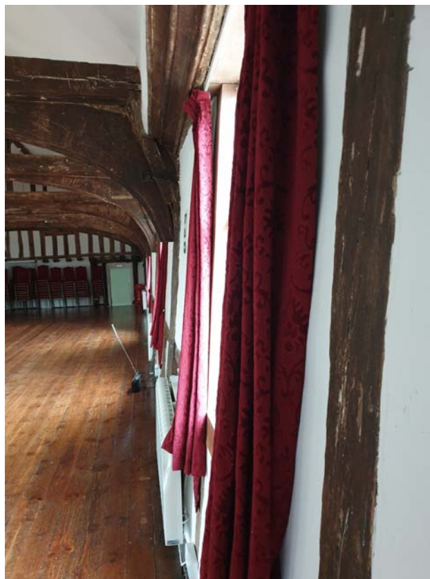
Photograph 116 – East wall bulging out, as seen from 'L1'
