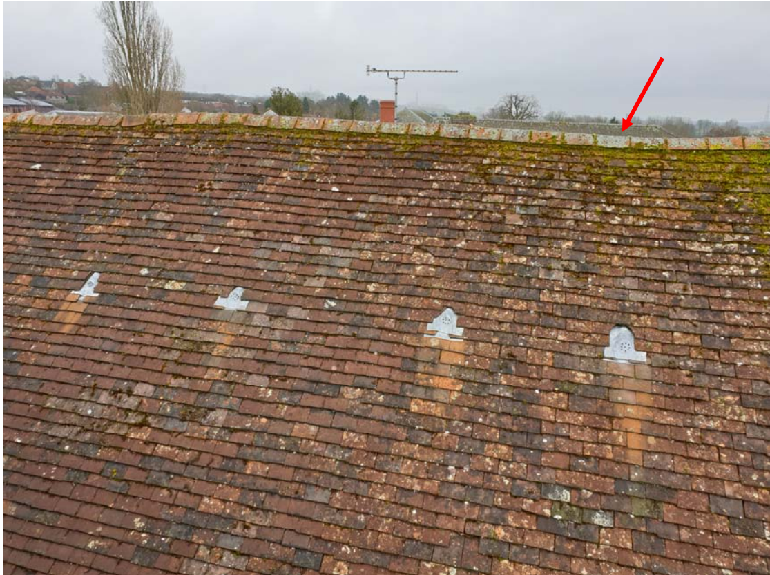
Photograph 05 – Undulations noted to the ridgeline of the roof over the south range of the Market Hall
