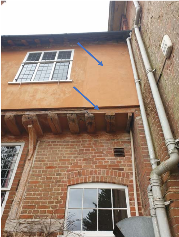
Photograph 99 – Sole plate repair and different nuance in the render to the south end of Old Town Hall’s west elevation
