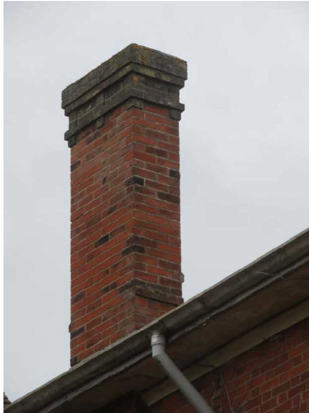
Photograph 129 – Cement-based mortar noted to the east chimney of the New Town Hall, as seen from the back courtyard
