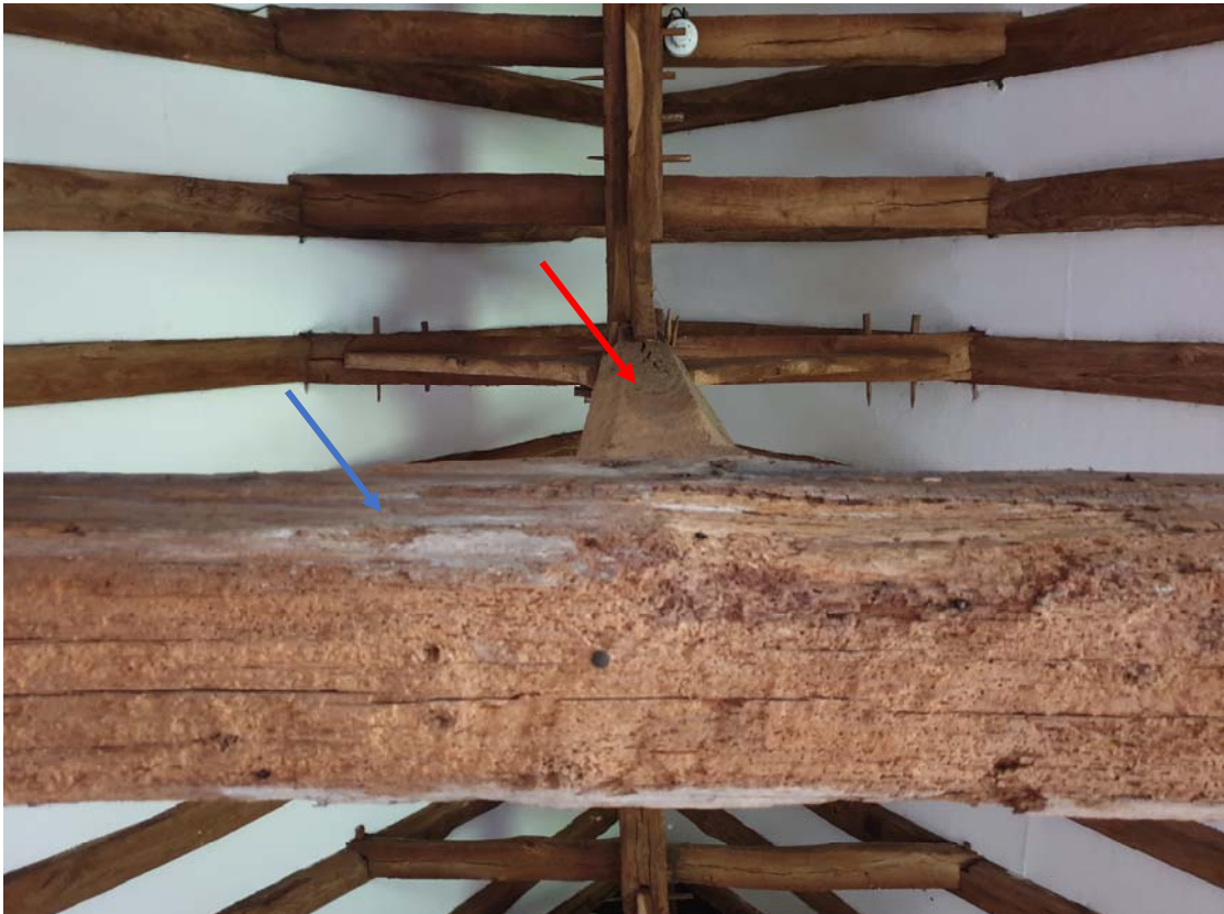
Photograph 50 – Crown-post (red) on timber tie-beam (blue) supporting the roof over Market Hall's middle range
