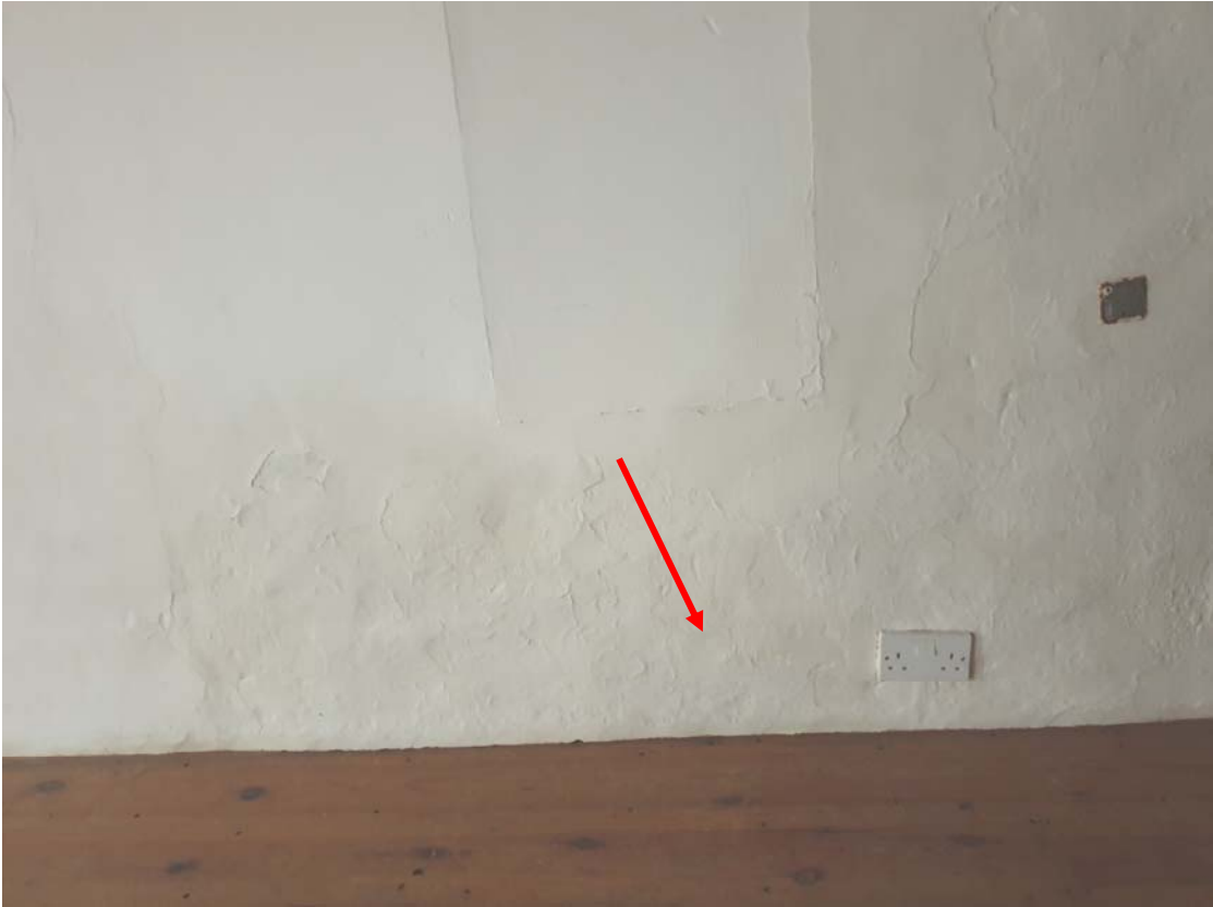
Photograph 108 – Historic dampness noted adjacent to the north fireplace in 'L4'
