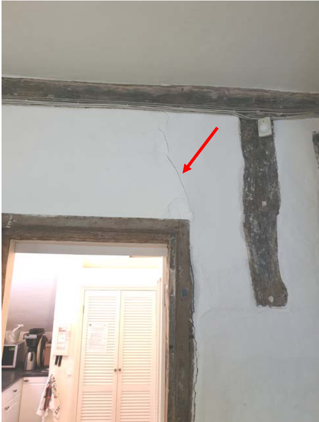
Photograph 80 – Live plaster and cracking noted above the door leading to 'R10'
