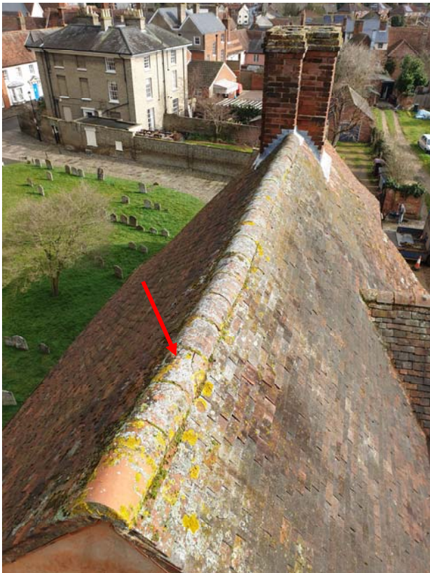
Photograph 18 – Fractured ridge tile to the Market Hall's middle range
