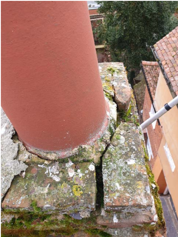
Photograph 88 – Damaged / missing flaunching to the north chimney of the Old Town Hall
