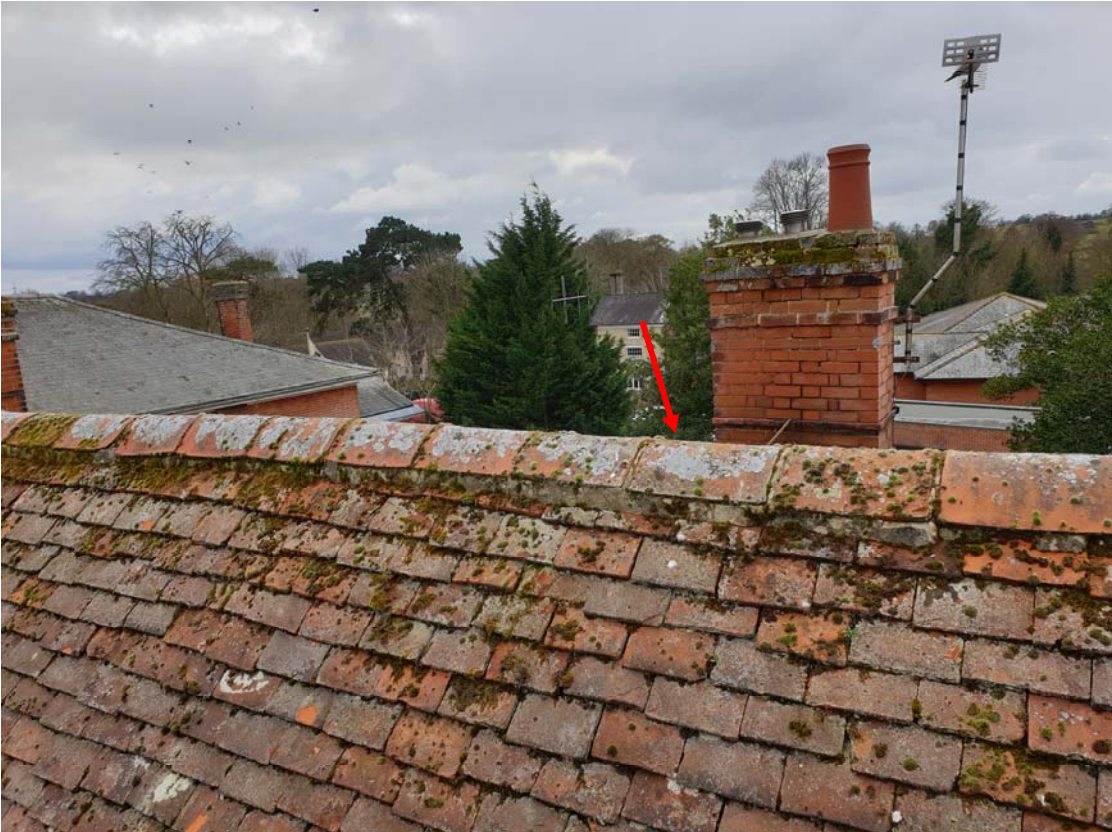
Photograph 84 – Undulations noted to the ridge beam over the Old Town Hall
