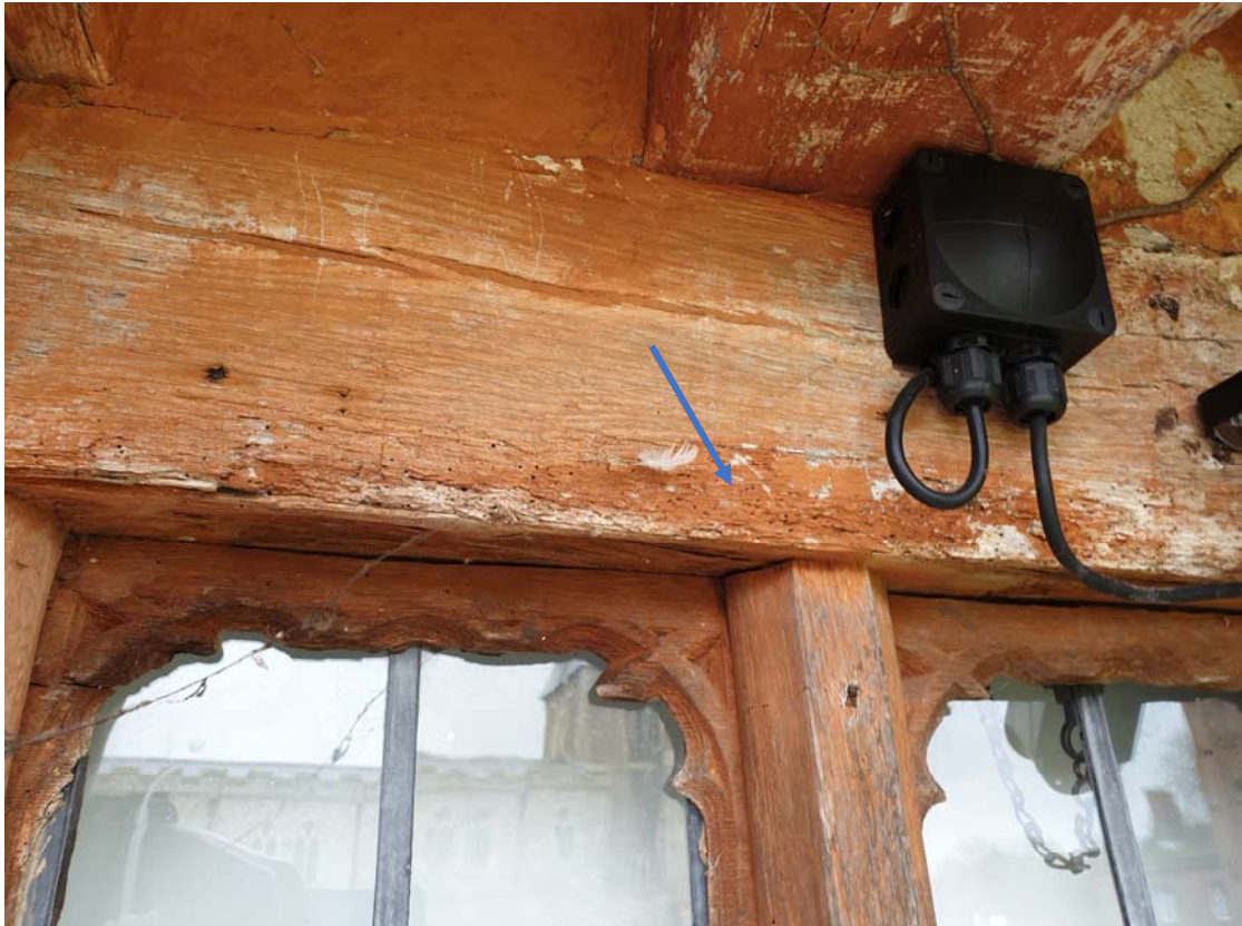
Photograph 33 – Local decay noted to the 1st floor west window of the middle range
