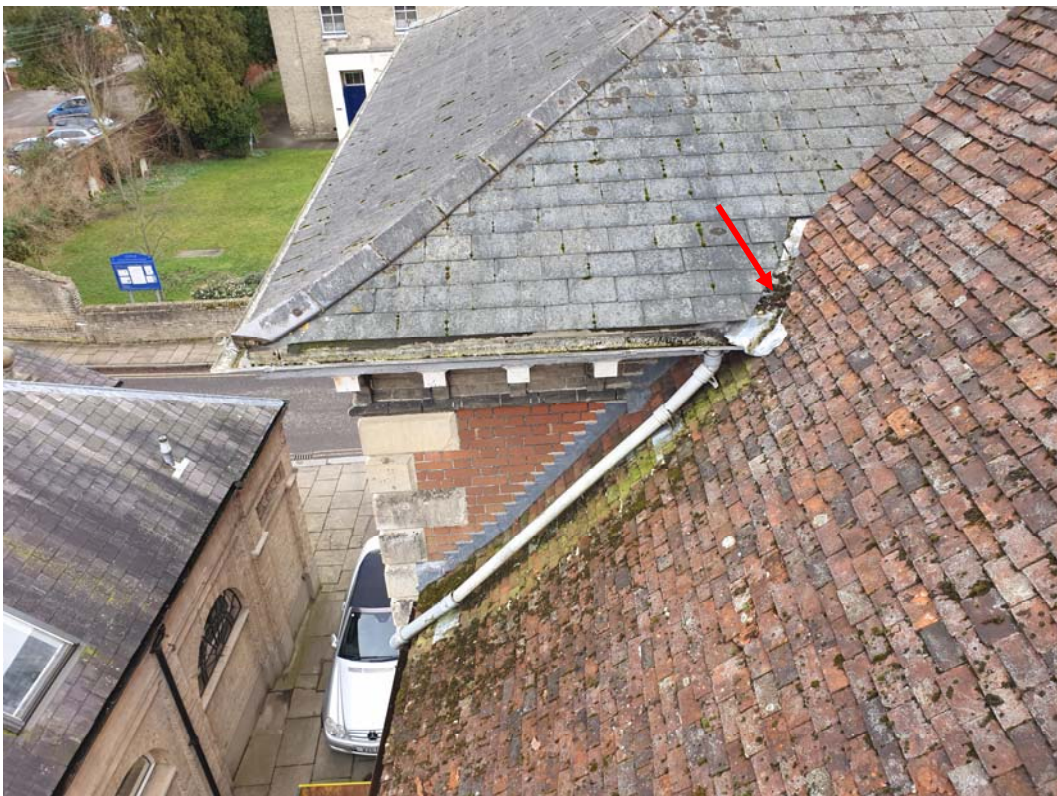
Photograph 86 – Moss build-up partially blocking the valley gutter at the junction between the Old Town Hall and New Town Hall
