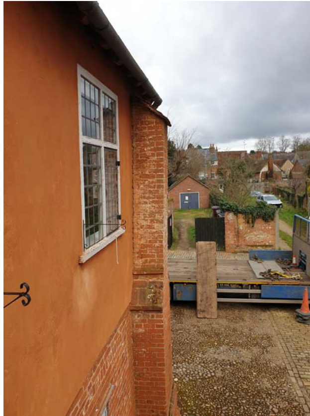
Photograph 47 – Out of plumb brickwork buttress to the south elevation of the east wing
