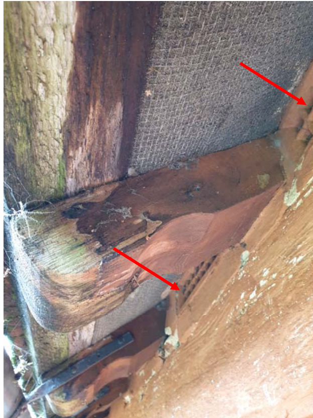
Photograph 27 – Air bricks noted to the eaves level of the middle range
