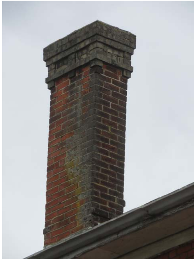
Photograph 125 – Central chimney that appears to be leaning slightly eastward
