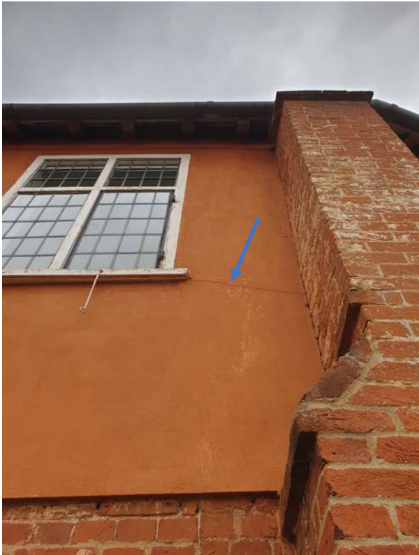
Photograph 49 – Diagonal cracking noted to the 1 st -floor windows (south elevation of Market Hall's east wing)
