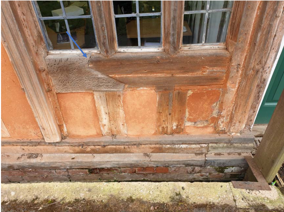
Photograph 37 – Scarf repair noted to the GF west window of the middle range
