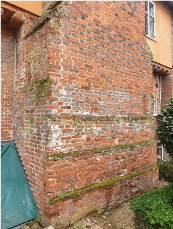
Photograph 97 – Few spalling bricks and moss vegetation noted to the base of the south chimney (Old Town Hall)
