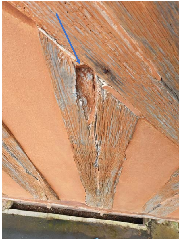
Photograph 29 – Decay noted to the exposed timber of the middle range
