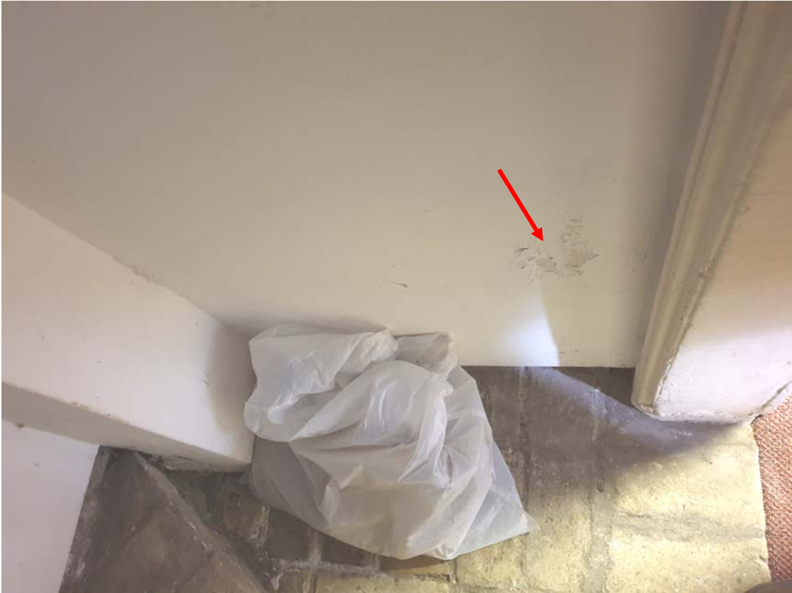
Photograph 83 – Poor decoration noted in the hallway leading to St. Mary’s Church
