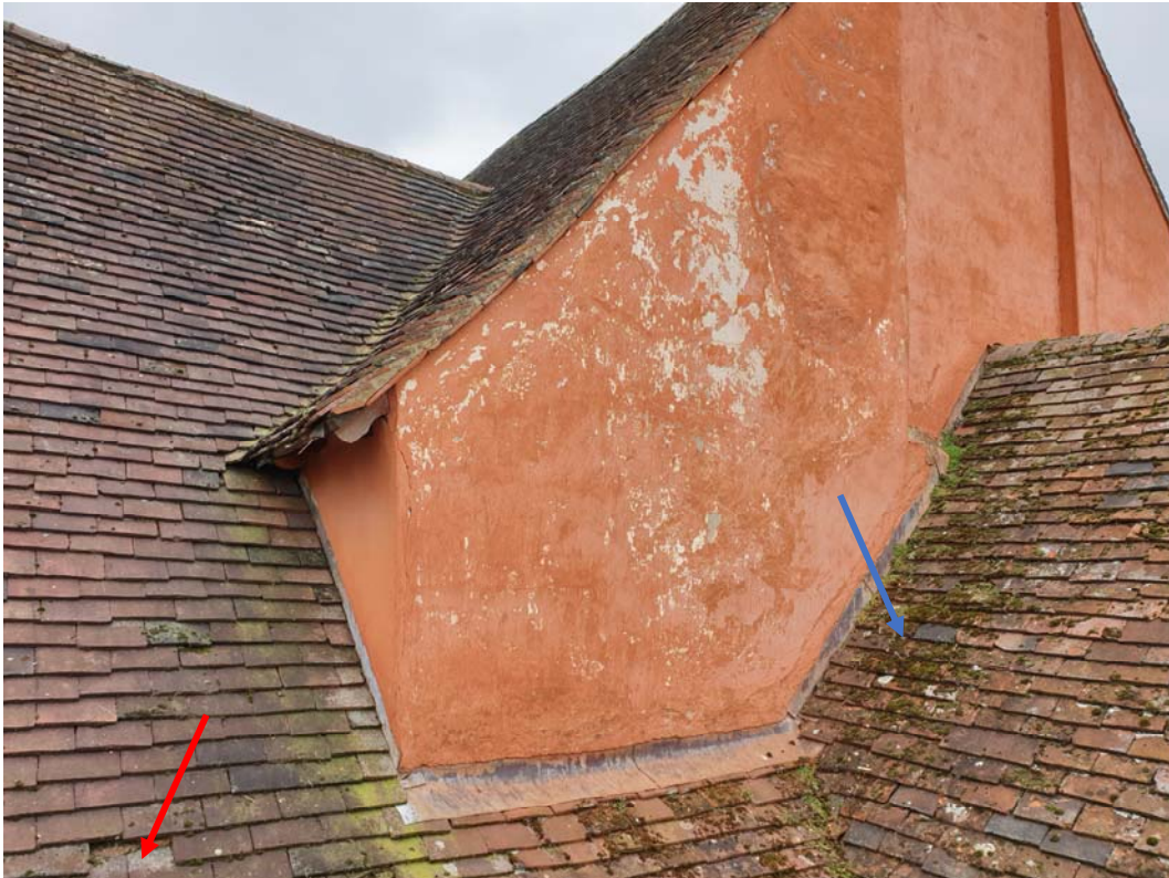
Photograph 85 – Moss vegetation (blue) and broken tiles (red) noted to the roof over the Old Town Hall
