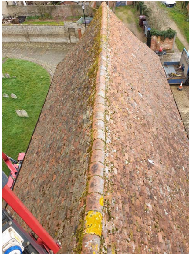
Photograph 41 – Roof over Market Hall's east wing, as seen from the cherry picker
