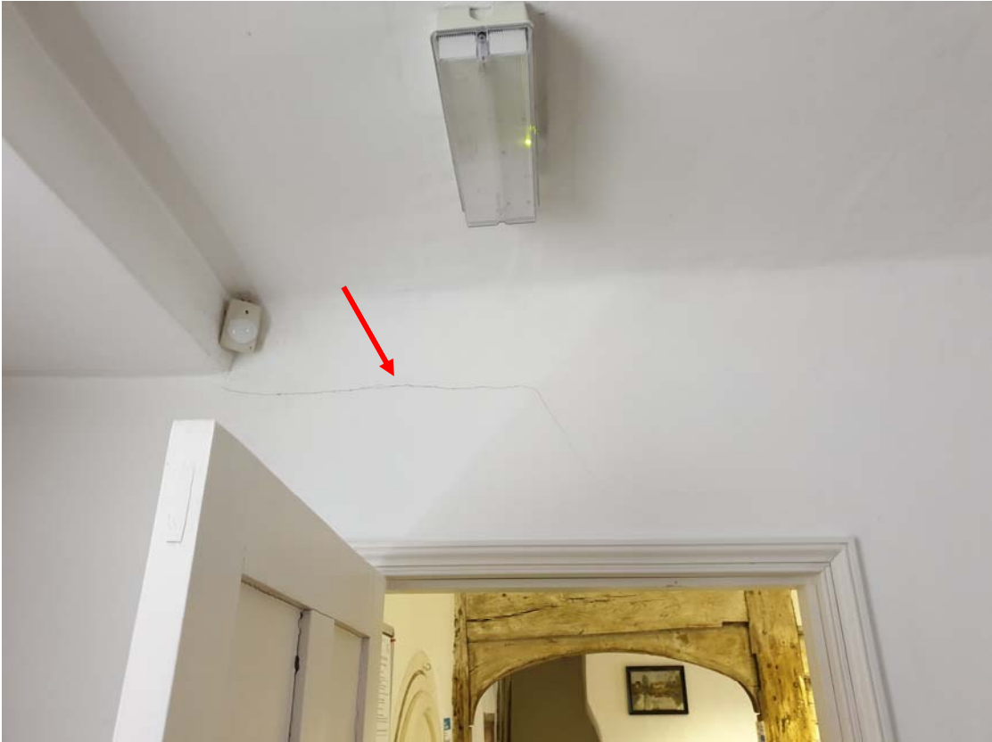
Photograph 77 – Horizontal hair-line crack noted in 'R7', above the door leading to 'R8'
