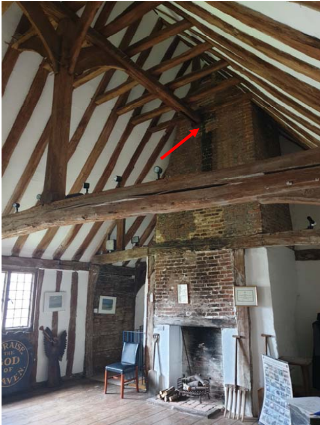
Photograph 51 – Cut back collar tie to the west face of the chimney breast in room ‘C1’
