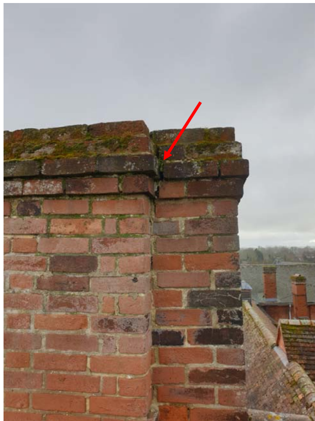
Photograph 22 – Minor separation crack to the middle range's chimney
