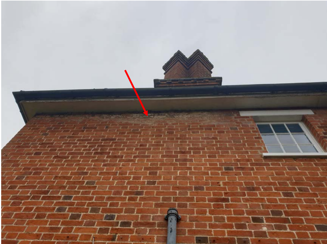
Photograph 15 – White stains at high-level – West elevation of Market Hall's west range
