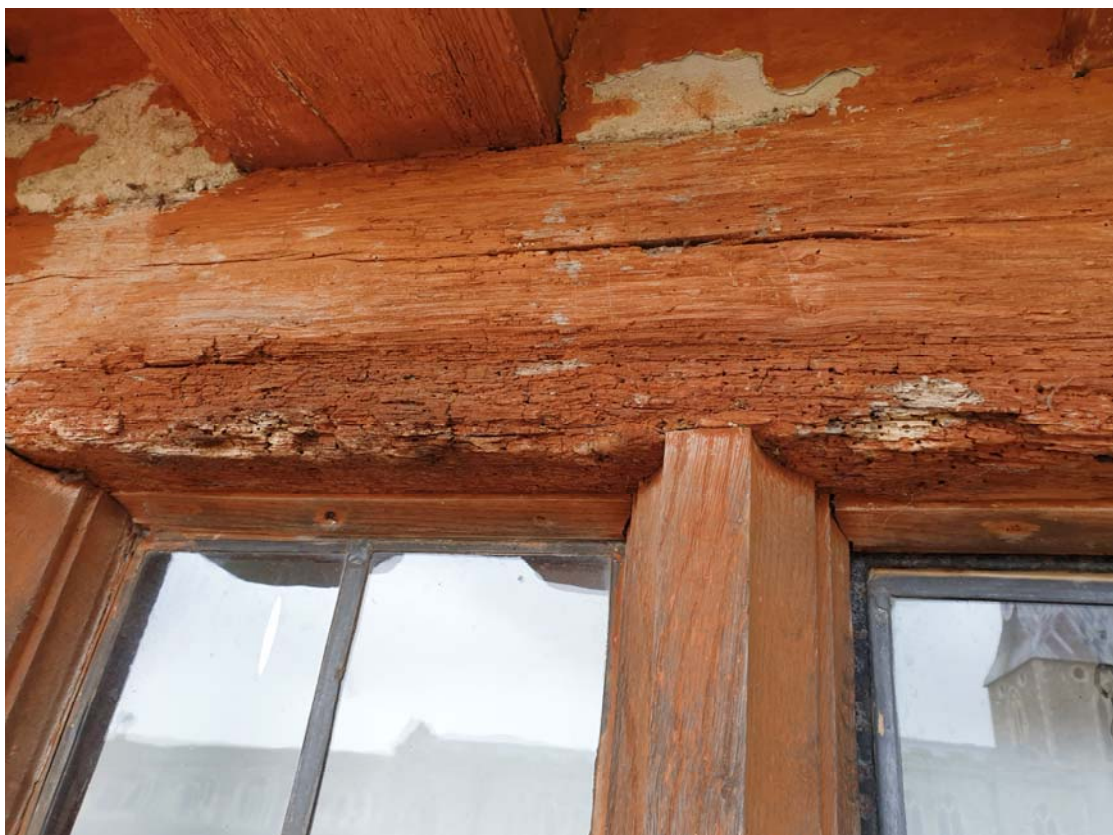
Photograph 32 – Rot noted to the 1 st -floor central window of the middle range
