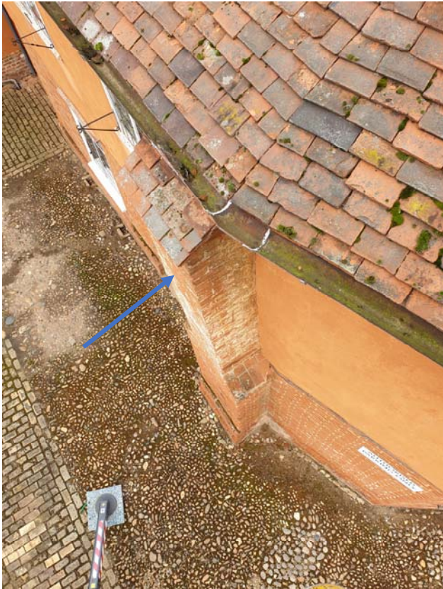
Photograph 45 – Brickwork buttress to the south elevation of the east wing (Market Hall)
