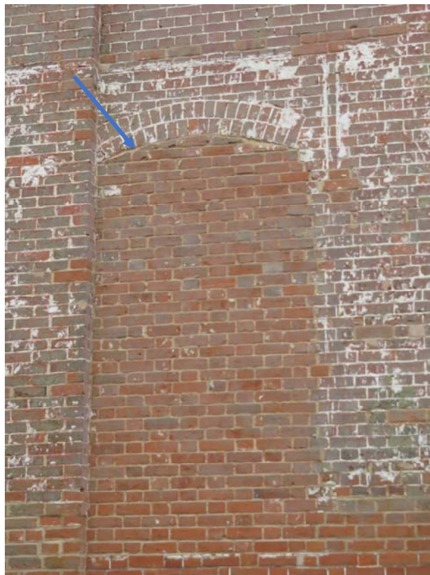
Photograph 130 – Evidence of historic door opening to the north elevation of the New Town Hall
