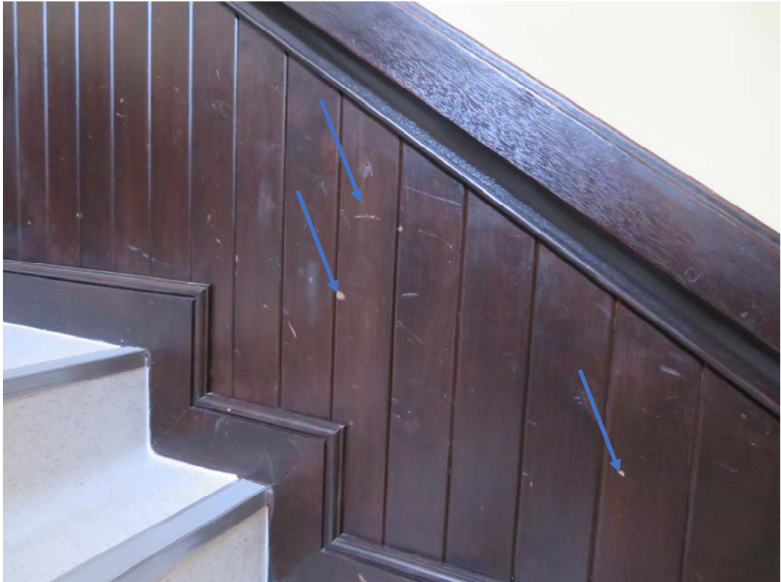
Photograph 139 – Timber joinery in need of redecoration noted to the stairs within New Town Hall
