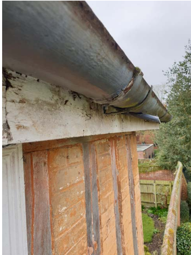
Photograph 11 – Paint flaking off at cornice level
