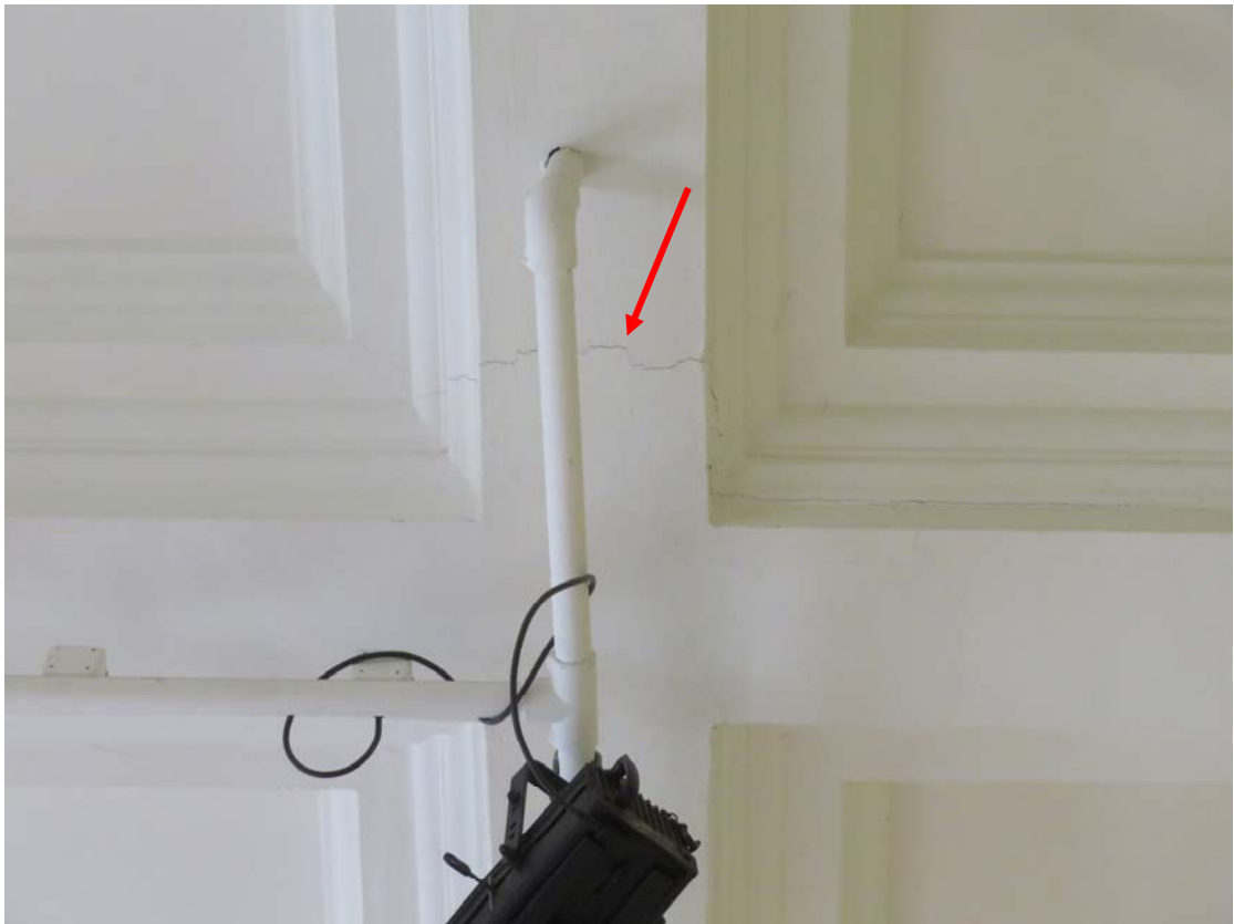
Photograph 136 – Cracks noted to the coffered beams noted in the Grand Hall
