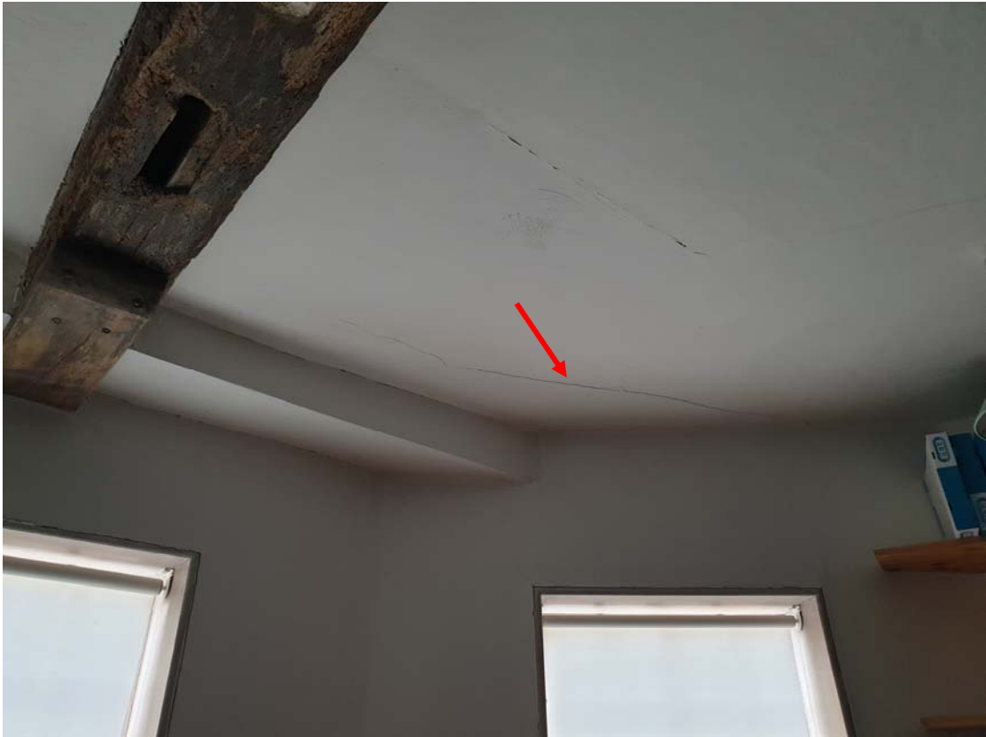
Photograph 73 – Cracks in the ceiling over 'R6' (east end)
