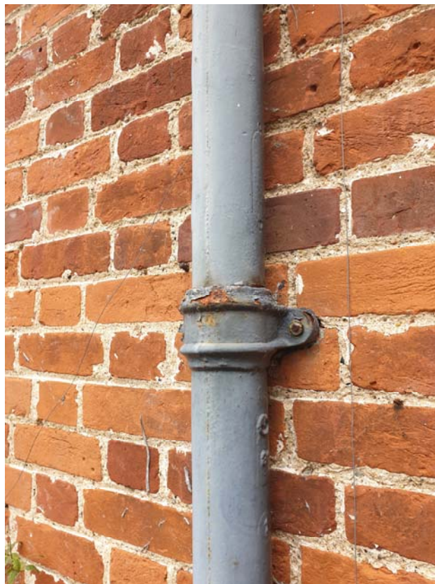
Photograph 14 – Cast iron downpipe in need of brushing and cleaning
