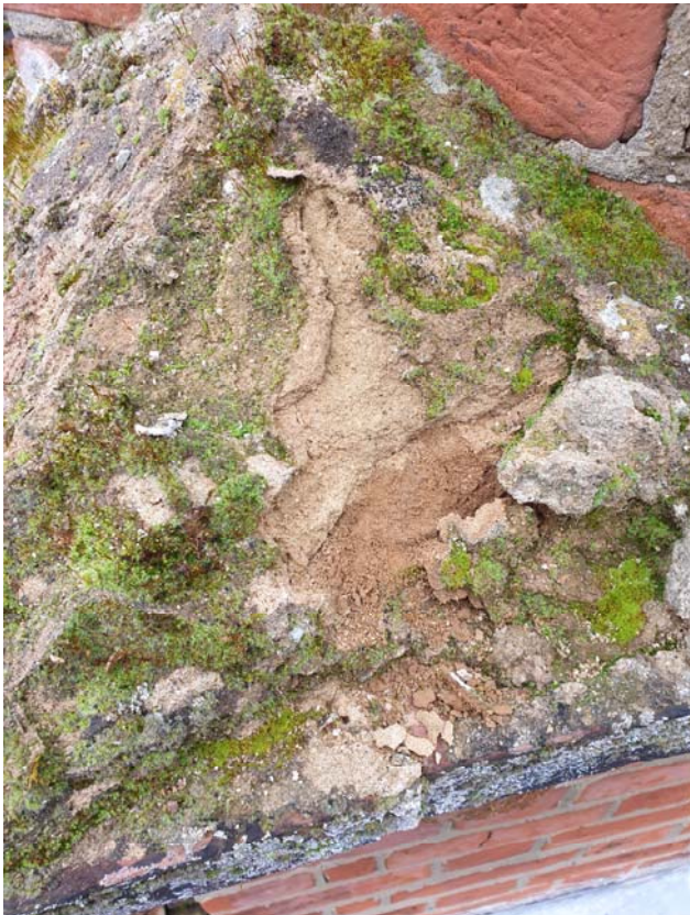
Photograph 08 – Delaminated flaunching to the South chimney
