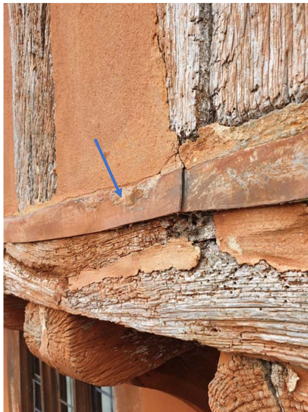
Photograph 30 – Lead flashings noted to the soleplates of the middle range
