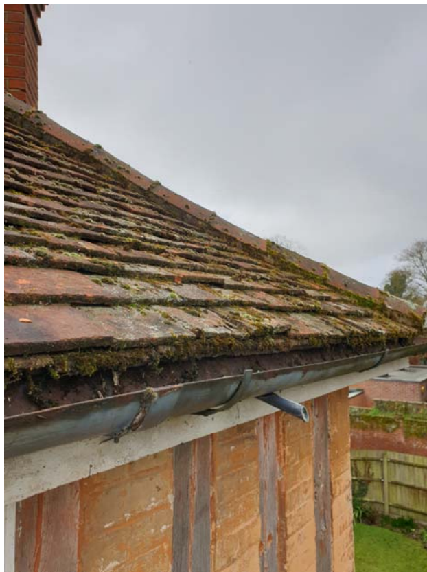
Photograph 10 – Metal gutters in need of brushing and cleaning
