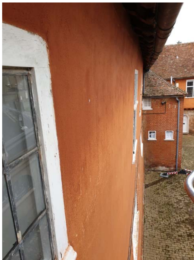
Photograph 90 – East elevation of the Old Town Hall bulging out at 1 st floor level
