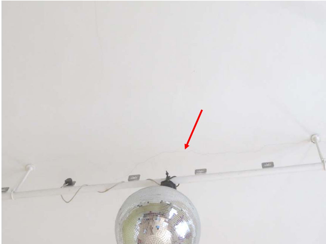
Photograph 137 – Crack to the flat ceiling, in line with the lighting rig, noted in the Grand Hall
