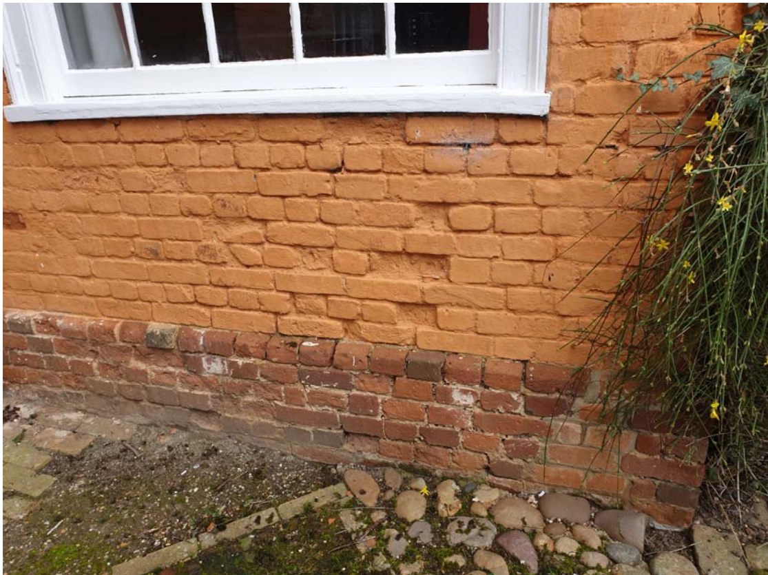
Photograph 92 – Delaminated bricks and eroded mortar joints noted to the north end of Old Town Hall's west elevation
