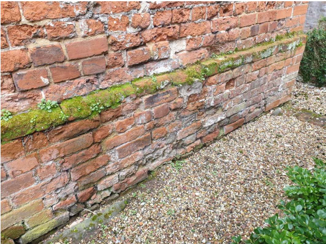
Photograph 98 - Few spalling bricks and moss vegetation noted to the base of the south chimney (Old Town Hall)
