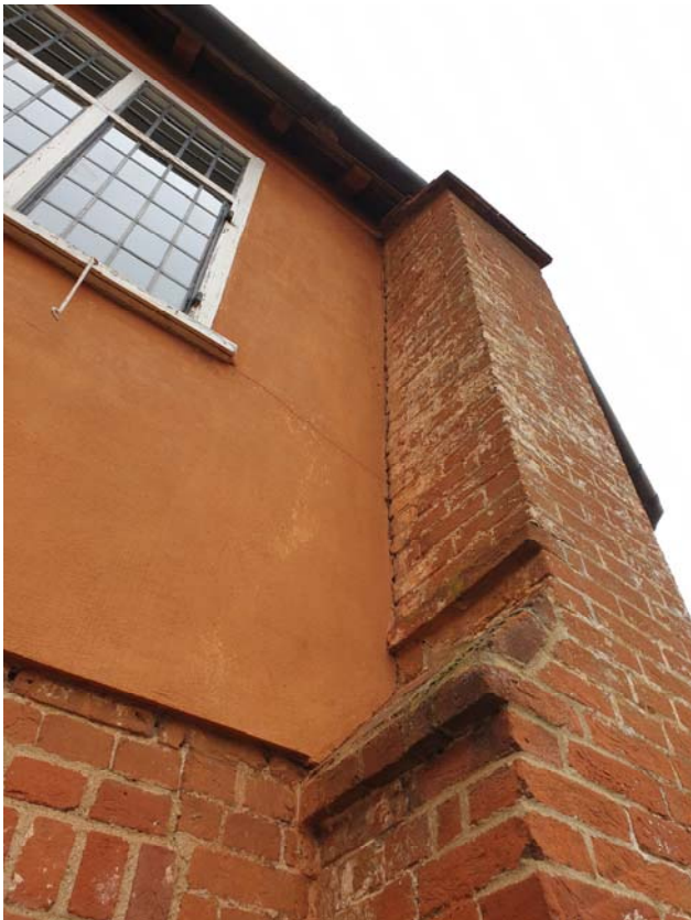
Photograph 46 – Movement noted to the buttress to the south elevation of the east wing
