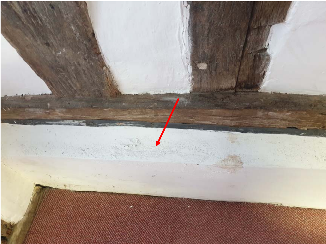
Photograph 82 – Dampness noted to the soleplate within room 'R11'
