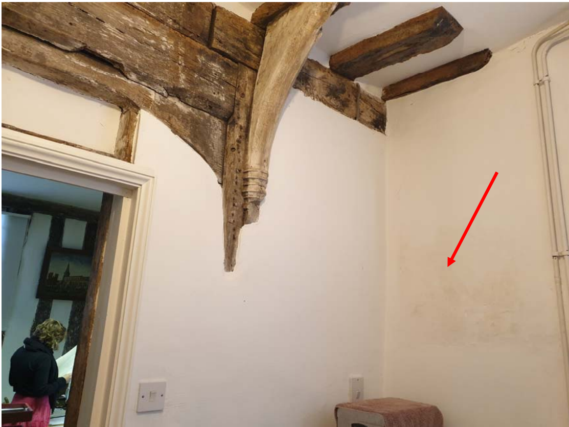
Photograph 104 – Historic damp stains noted in 'R10'
