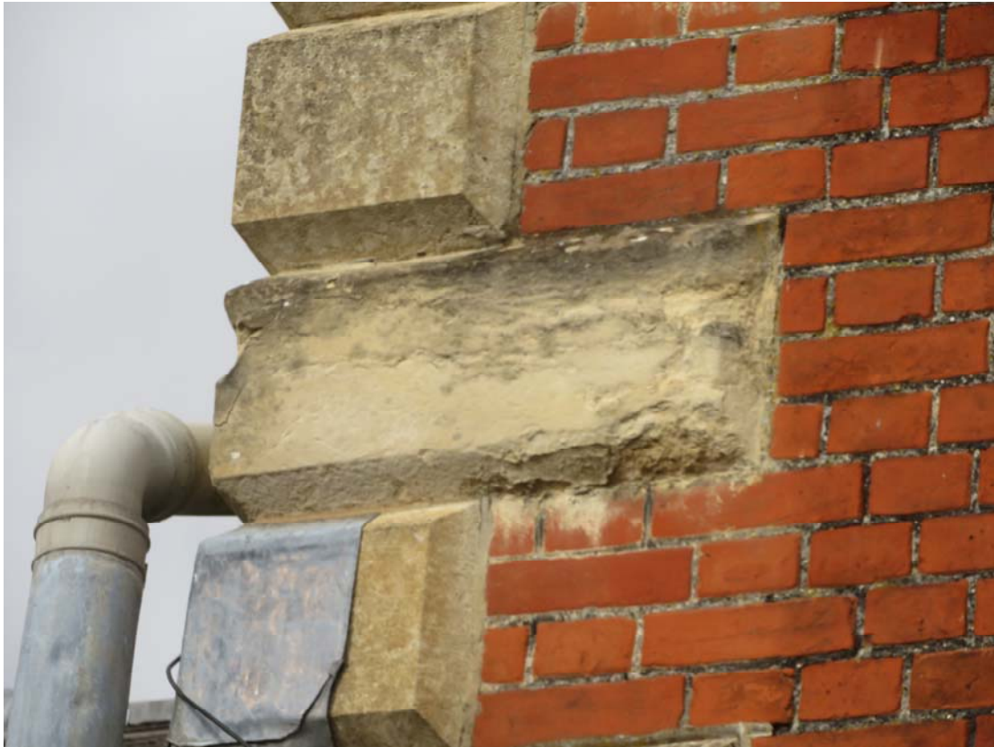
Photograph 119 – Detritus and pollution stains to the stone quoins of New Town Hall
