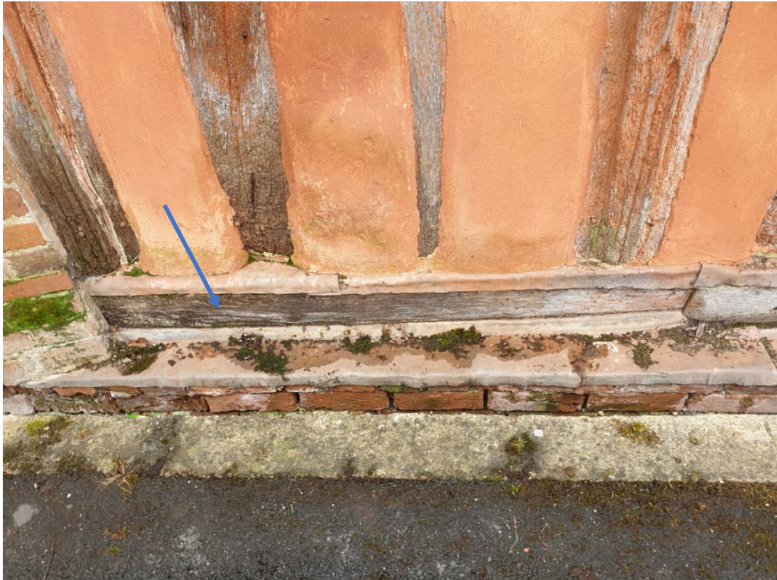
Photograph 39 – Dampness noted to the east end of the soleplate (middle range)
