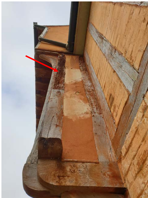
Photograph 36 – Decay noted to the north-west corner post of the middle range
