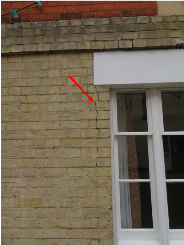
Photograph 121 – Cracking noted in line with the lintel to the centre window to the front elevation of the New Town Hall
