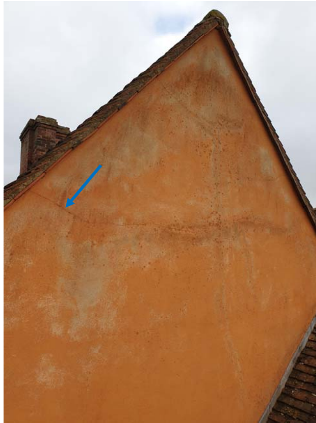
Photograph 25 – Minor cracking in the render to the west gable of the middle range
