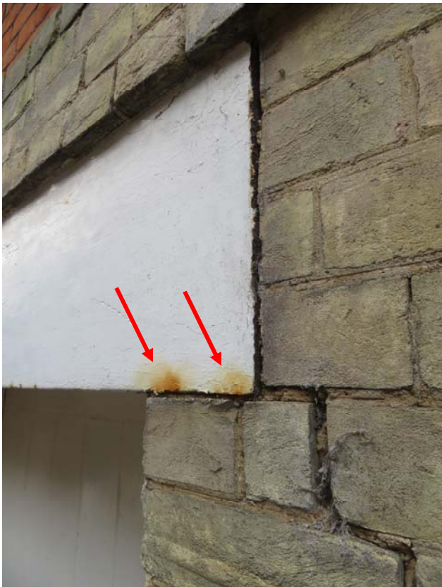
Photograph 124 – Corrosion to the base of the lintel, to the east elevation of the New Town Hall
