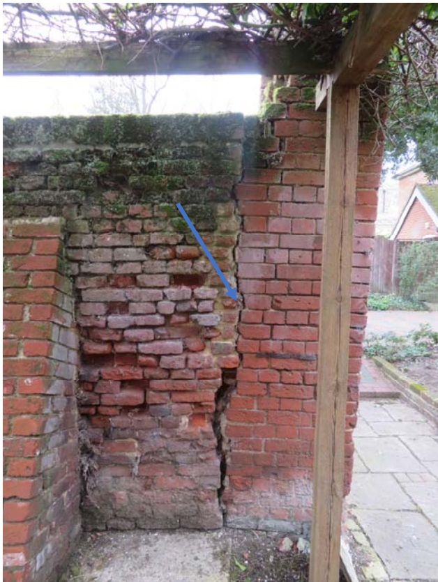
Photograph 134 – Movement noted to the south-east corner of the old Tudor kitchen
