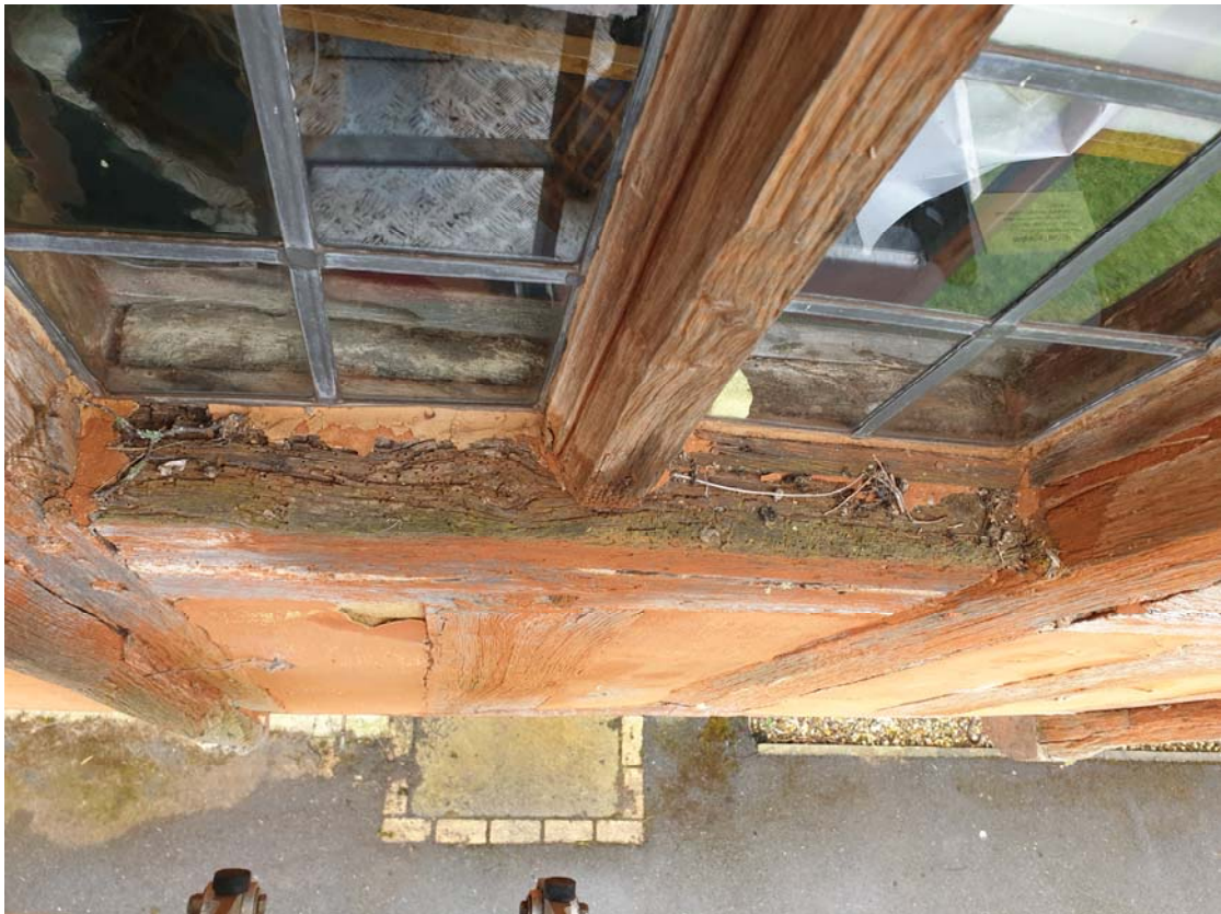
Photograph 34 – Decay noted to the sill of the 1st floor west window (middle range)
