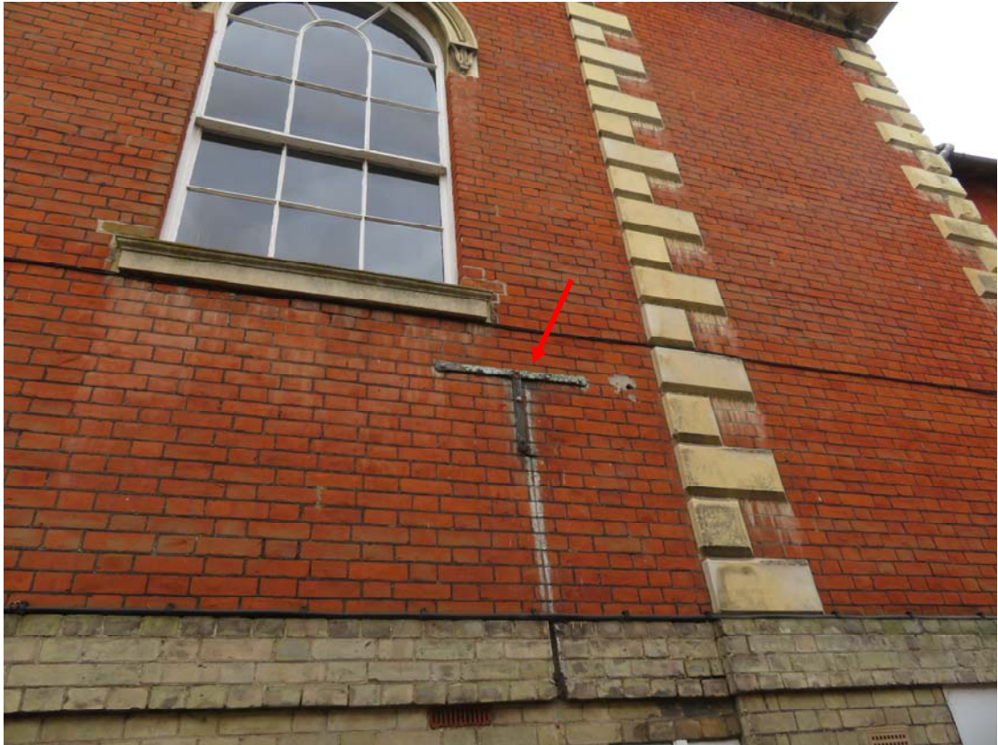
Photograph 123 – Iron bracket noted to the east elevation of the New Town Hall
