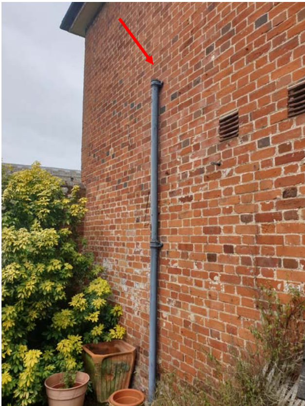
Photograph 16 – Missing section of downpipe to the west elevation of the Caretaker's range
