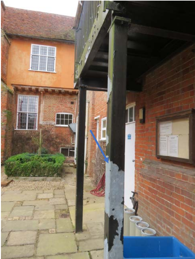
Photograph 131 – Galvanised steel escape stair showing signs of failing finishes
